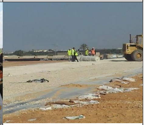
Gravel filter in Johr Al Dik landfill
